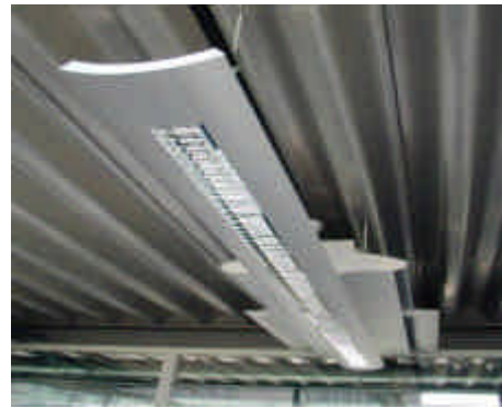
Stainless steel profiled decking and lighting/air distribution units
