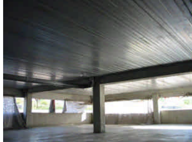
Under site view of the finished slab. False ceiling will be provided for services.
