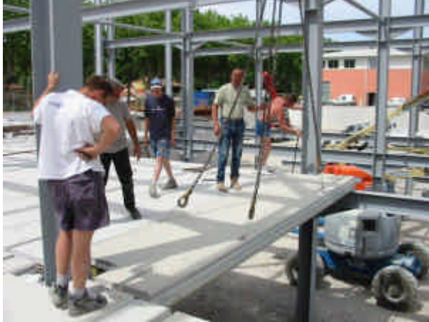
Positioning of element on site. Fast construction process – intensive use of steel elements
